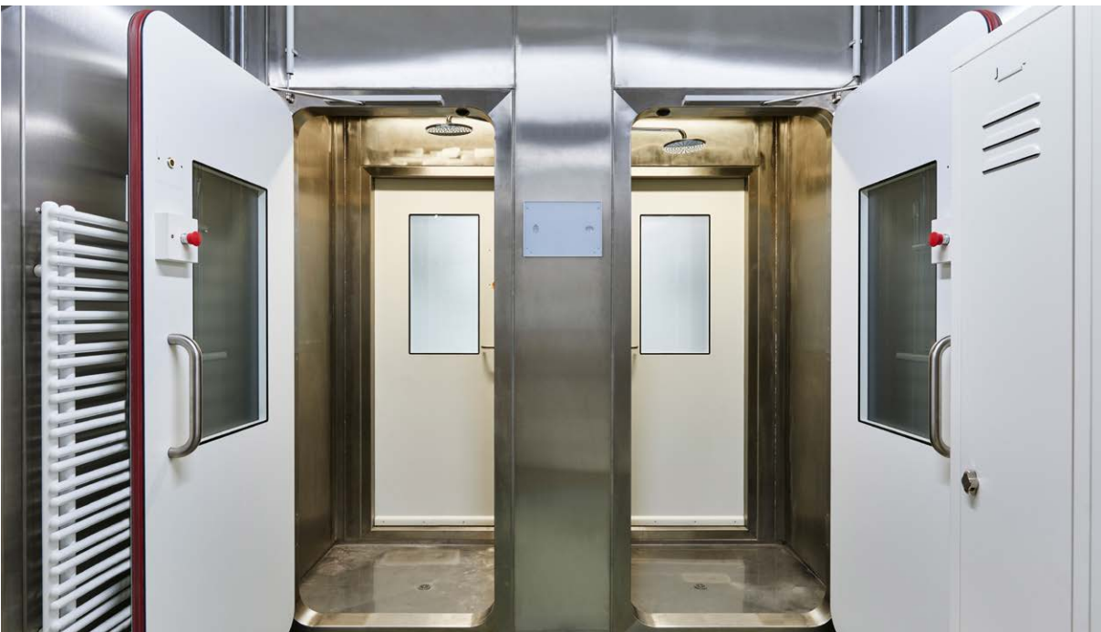
Figure 2: Entrance to Laboratory via Personnel Showers
